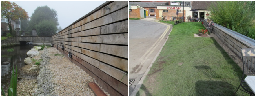
At Marlborough a flood alleviation scheme was jointly funded by the Environment Agency, Wiltshire Council and Marlborough Town Council.
