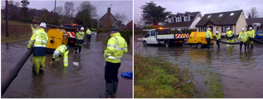
Wiltshire Council's staff and contractors responded to many requests for assistance during the flooding in 2014.
