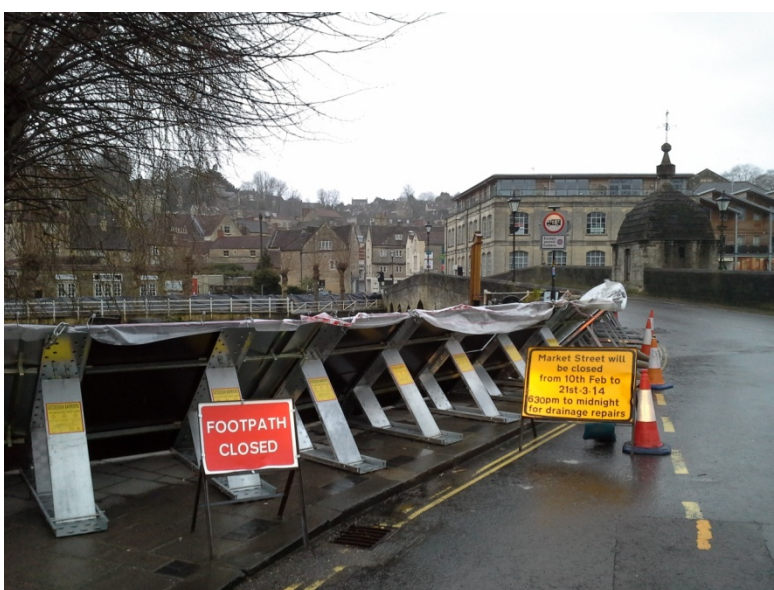
In 2014 Wiltshire Council worked with the Environment Agency to install temporary flood barriers to help protect Bradford on Avon from flooding from the Bristol Avon.
